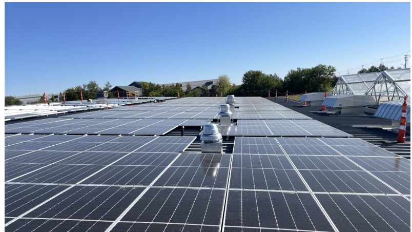
Roof top photovoltaics produce enough energy year round to power the building. The production greenhouses to the right allow students to study crop issues including plant growth, water, and weeds.
